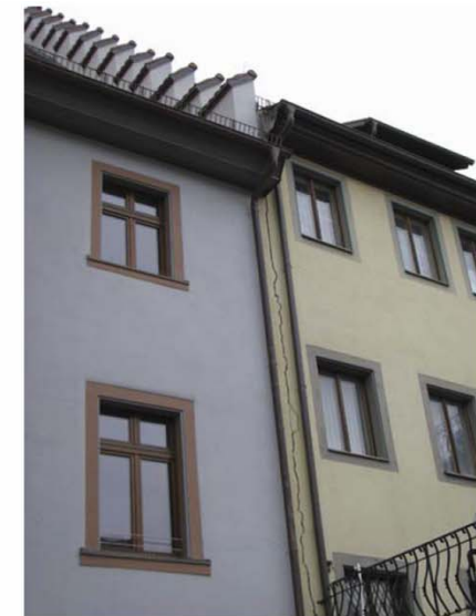
Fig. 3 Vertical open crack in the city centre that cuts two buildings from the ceiling to the roof
